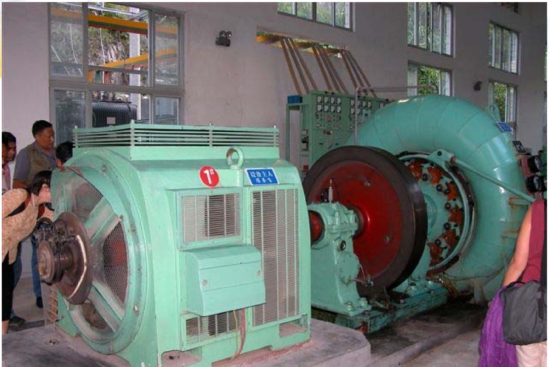
360 kW Small Hydro Unit in Zhejiang Province, China (Total Plant Capacity 1.18 MW)
